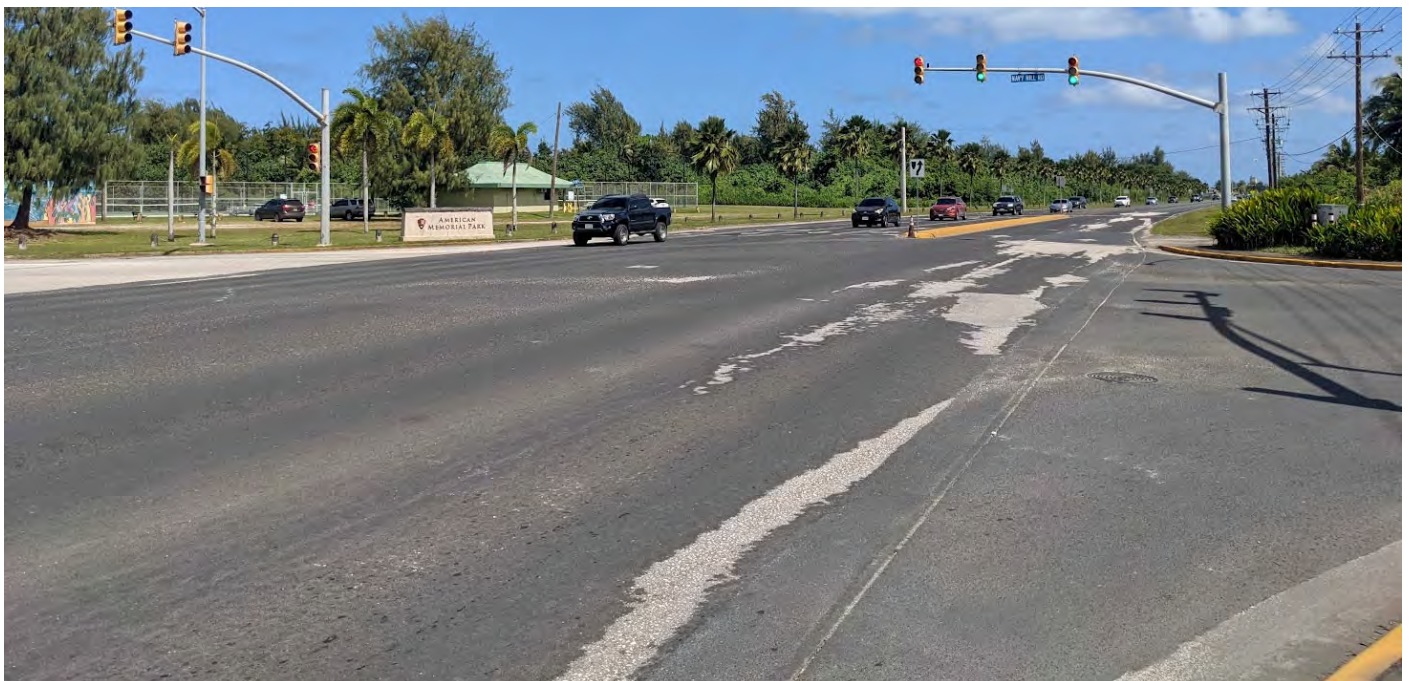
Photo 6-47 Existing Condition: Missing Crosswalk at Route 38/Route 39 Intersection – Northbound View
