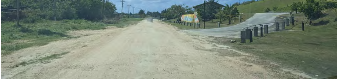
Photo 6-2 Example of Poor Pavement & Striping Conditions at the Intersection of Route 38 & Route 30 (Saipan)
